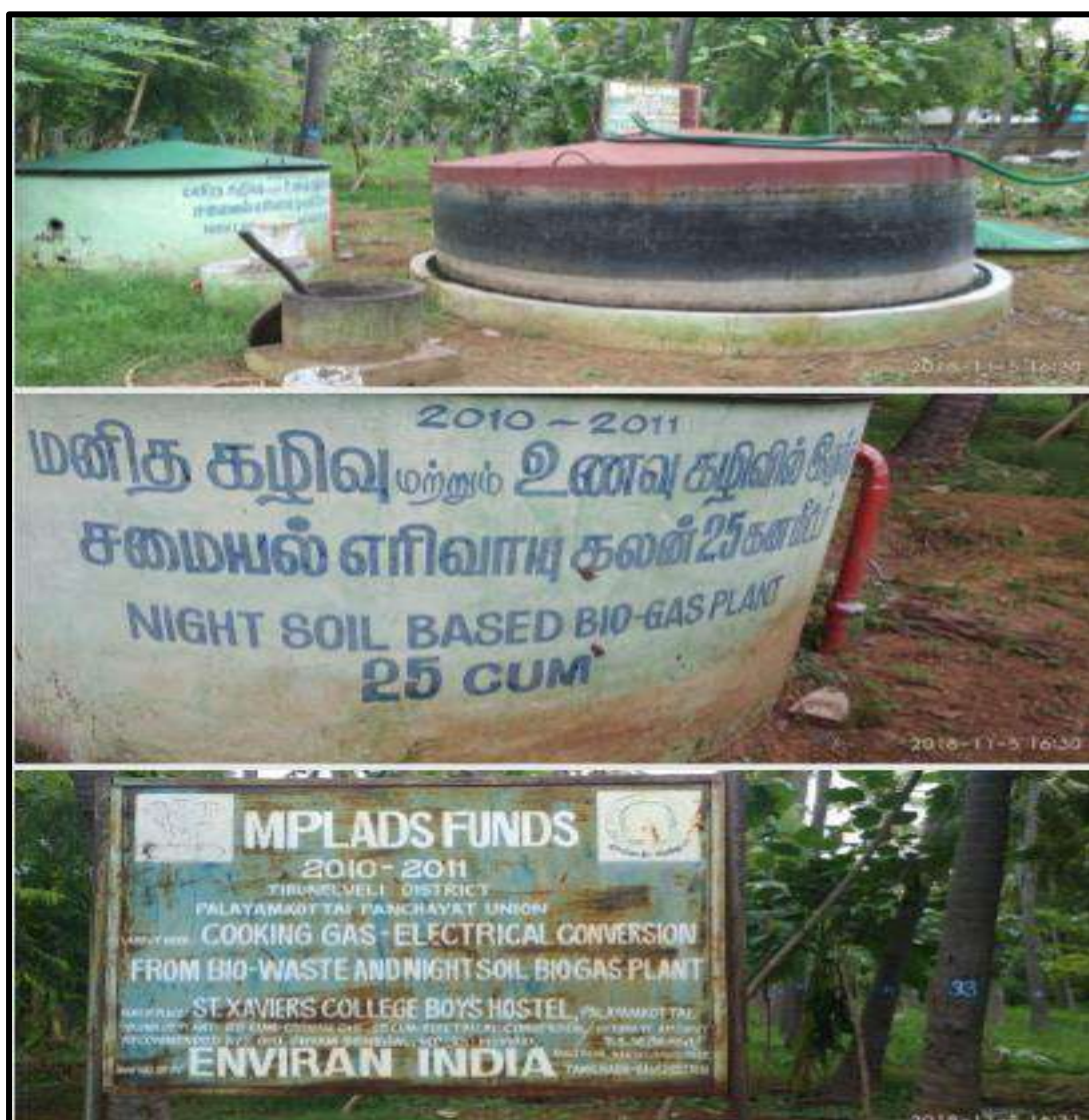
Biogas plant set up in the St. Xavier's College, Palayamkottai – 627 002, Tamilnadu.
